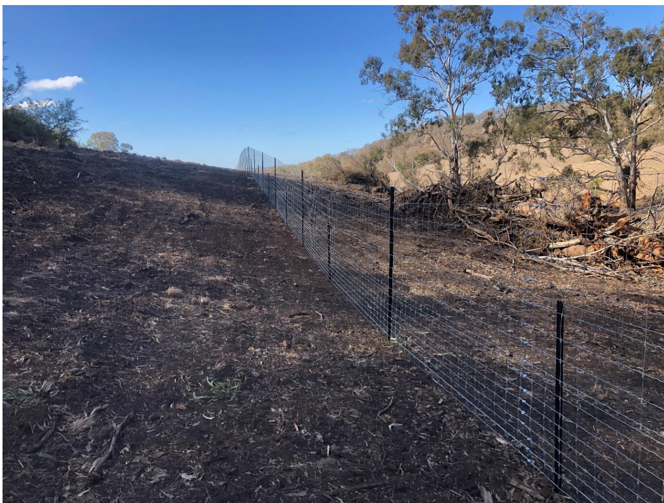
Figure 5. Prior to erecting this deer exclusion fence, the fence line was cleared (i.e. trees pushed aside) and levelled by a bulldozer.
