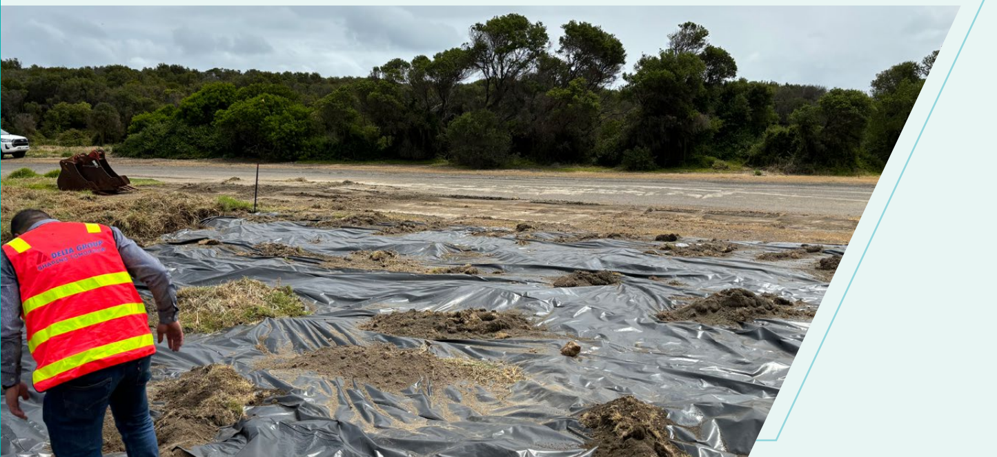
Photo: Heavy-duty plastic used to cover the test pit between testing and remediation works Credit: SMEC Australia Pty Ltd.
