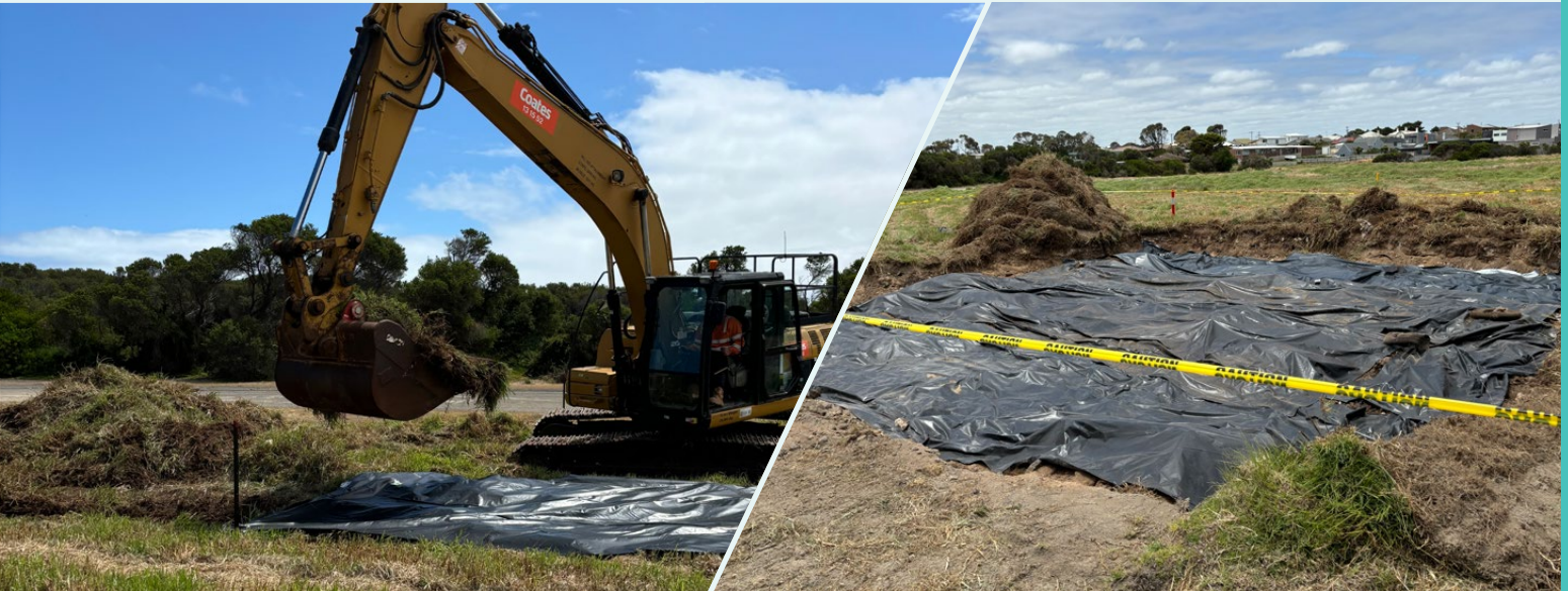
Photo: Securing the test pit cover with stockpiled topsoil Credit: SMEC Australia Pty Ltd.
